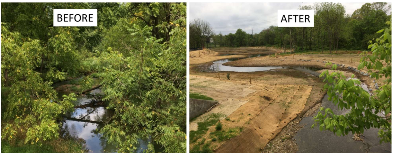
(Stream "restoration" in Blohm Park, Gaithersburg at Watkins Mill Rd. over Whetstone Run at the same location. Note the stream bank armor-plating on the right. (Left on 9/3/2020; right on 5/03/2021); by K.Bawer)
