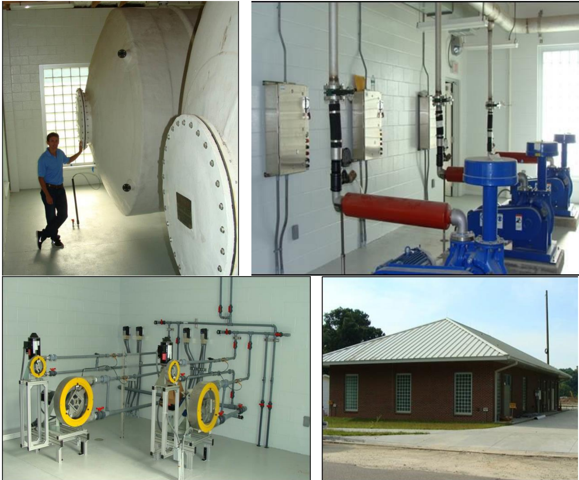
Figure 9. Photos from the Upper Lake Lafayette Nutrient Reduction Facility
