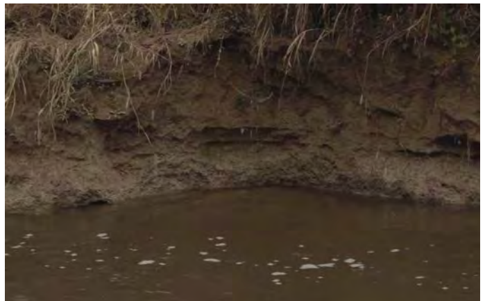
Collapsed banks and steep drops between the shoreline and water surface are signs of shoreline erosion. ( Will Parson )
