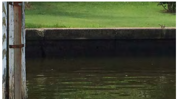
A deteriorating concrete bulkhead in Harford County. (Rebecca Swerida)
