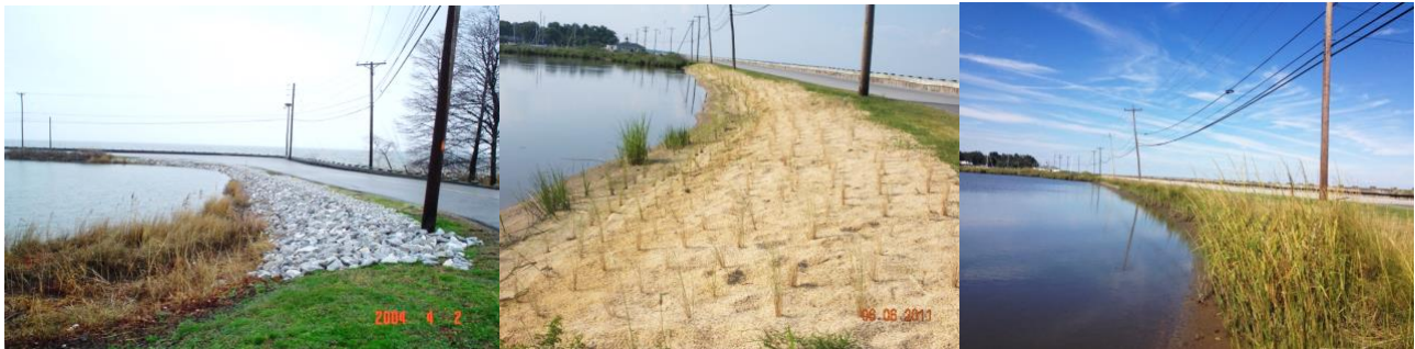
Figure 6. Pictures of the BayLand Engineering Green Riprap installation at Gibson Island at various stages of completion. From left to right, the images show the after riprap construction (2004), after filling and planting (2011), and one year after planting (2012). Images provided by BayLand Consultants & Designers, Inc.
