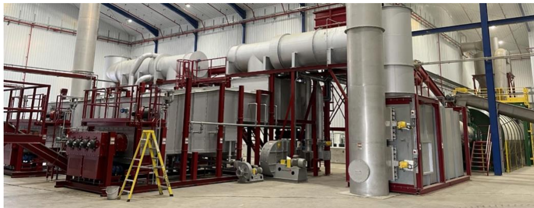
Figure 15. Dual 40 ton/day/Gasifiers (Photograph Credit – Earthcare, LLC ).
