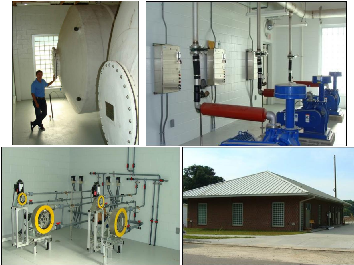
Figure 11. Photos from the Upper Lake Lafayette Nutrient Reduction Facility
