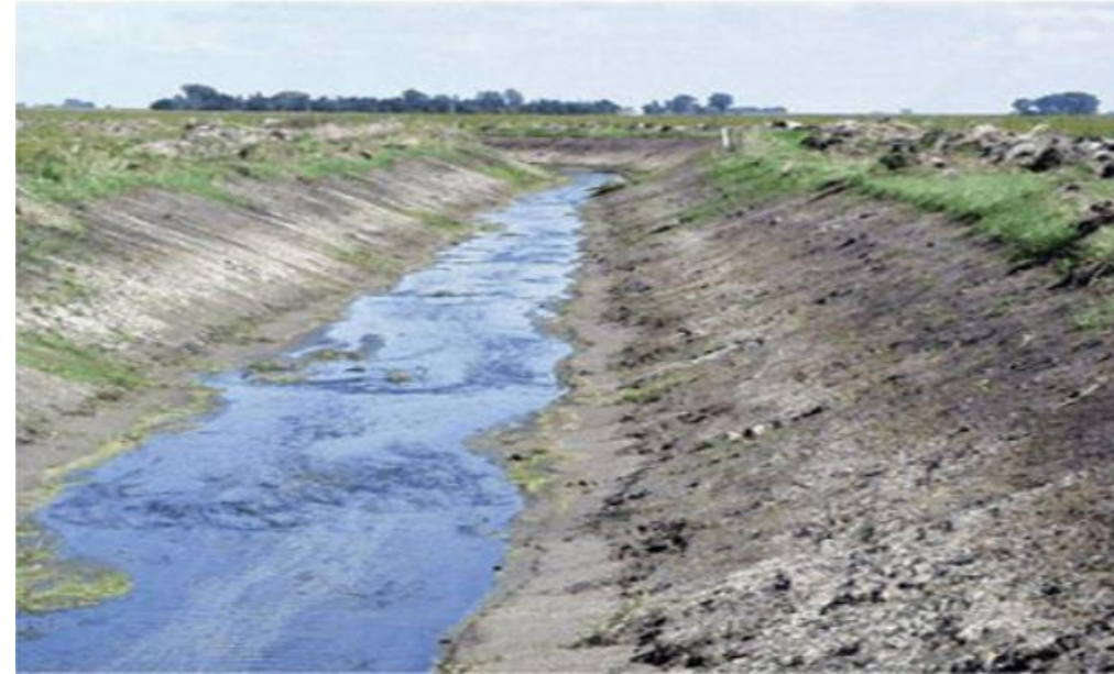
Traditional drainage ditch after a cleanout. Source: Ohio State University Extension, https://agditches.osu.edu/image-galleries/drainage-channels
