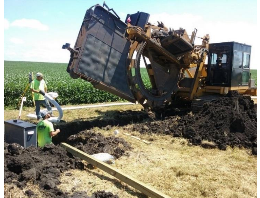
Figure 14 in report. Installation of a saturated buffer. Source: USDA ARS 2015. Photographer: Dan Jaynes.
