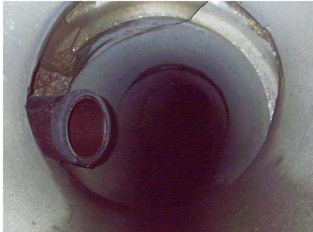
Sewer Lateral Connected to the Storm Drain System (Walch, DelDOT)
