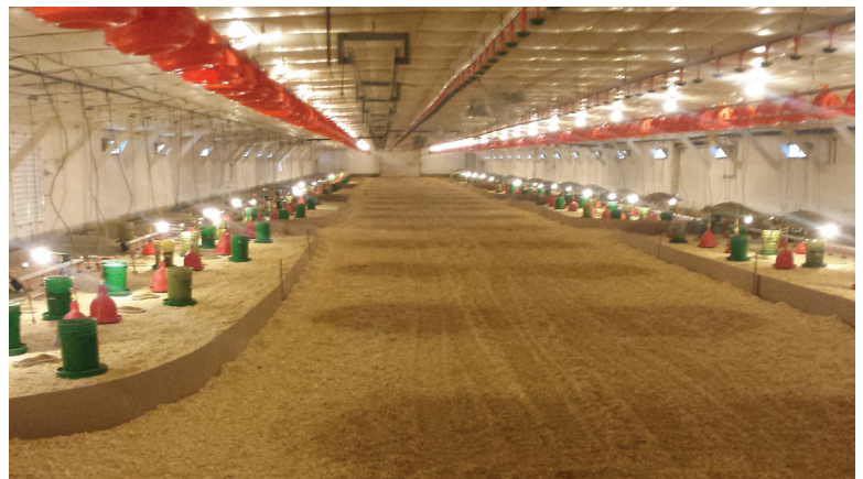
A brooder turkey barn is equipped with under-the-floor pipes that carry heated water from the bio-burner. (Photo: Glenn Rodes)
